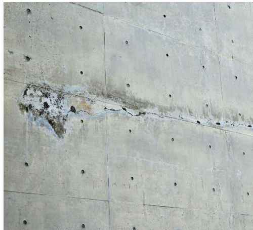
Figure 1. Impediment to integration due to the occurrence of cold joints.
